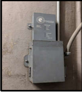
Blow Down Box: OFF
