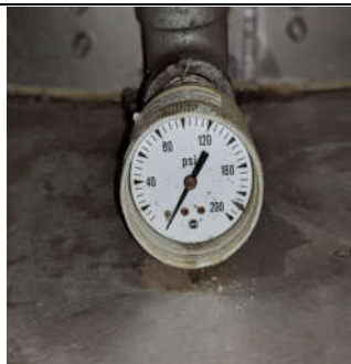
Pneumatic pressure gauge. Should be at 0
