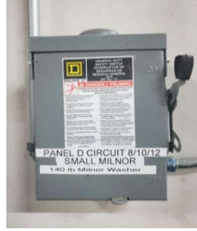
Electrical Disconnect: ON
