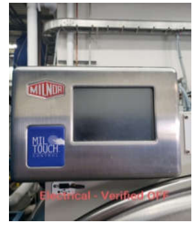
Electrical Panel: OFF
