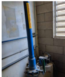
2nd Source of Geothermal Shutoff
