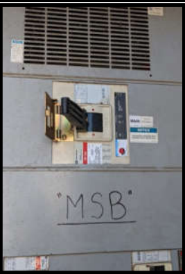
Outside Electrical Panel: Main Switch.
