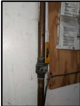
Air Line #2: 2nd source of shut off
