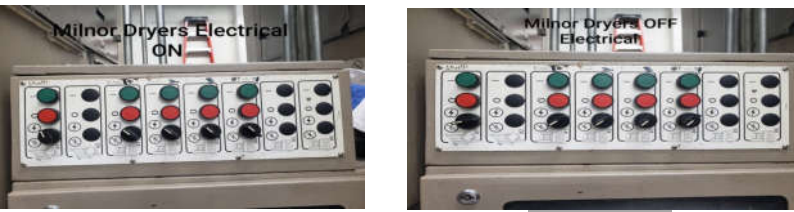
Electrical Disconnect: ON
