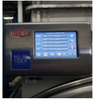
Electrical Panel: ON
