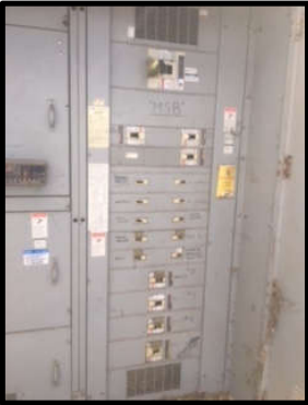
Electrical Panel located by front door. MAIN switch
