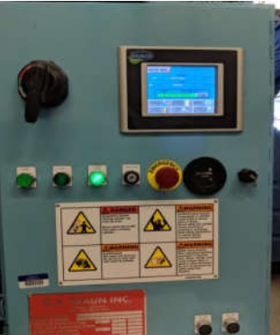
Electrical Panel ON
