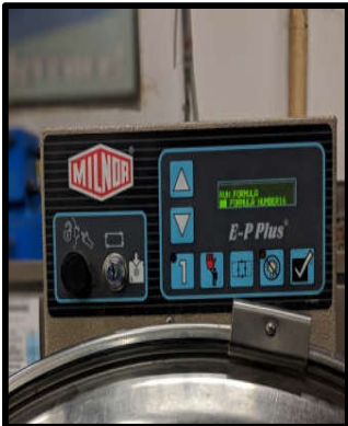
Electrical Panel: ON
