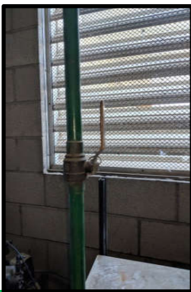
Air Line #1: 2nd source of shut off
