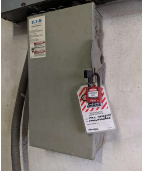
Electrical panel w/LOTO
