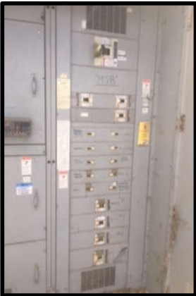
Electrical Panel located by front door. MAIN switch
