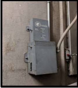
Blow Down Box: ON
