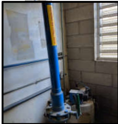
2nd Source of Geothermal Shutoff
