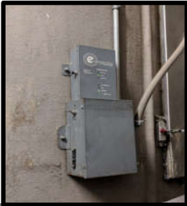
ELECTRICAL: Blow Down Box
