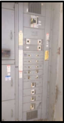
Electrical Panel located by front door. MAIN switch
