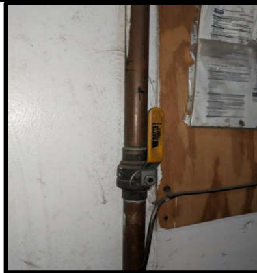
Air Line #2: 2nd source of shut off
