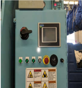
Electrical Panel OFF
