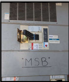
Outside Electrical Panel: Main Switch.
