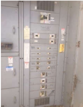
Main Electrical Panel located by front door. Switch marked 600 Washer
