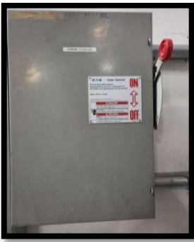
Electrical Disconnect: ON
