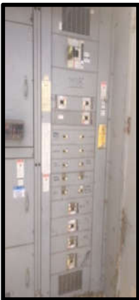
Electrical Panel located by front door. MAIN switch
