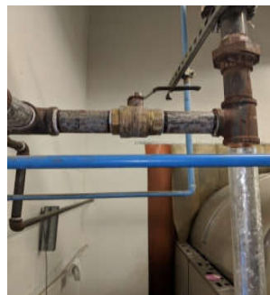
Steam : 2nd source of shutoff
