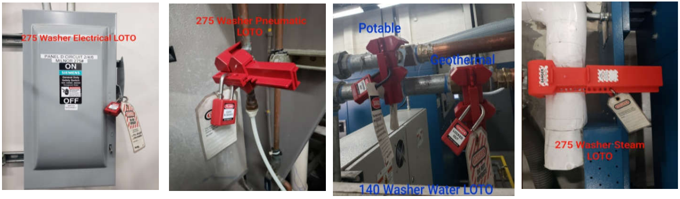
Electrical: LOTO Pneumatic: LOTO Water: LOTO Steam: LOTO
