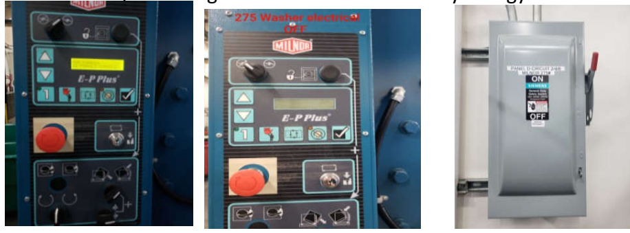
Electrical Panel: ON Electrical Panel: OFF Electrical Disconnect: ON Electrical Disconnect : OFF
