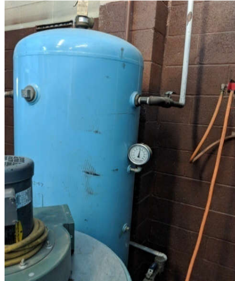
Air cylinder to verify de-energization
