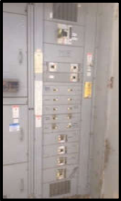
Electrical Panel located by front door. MAIN switch
